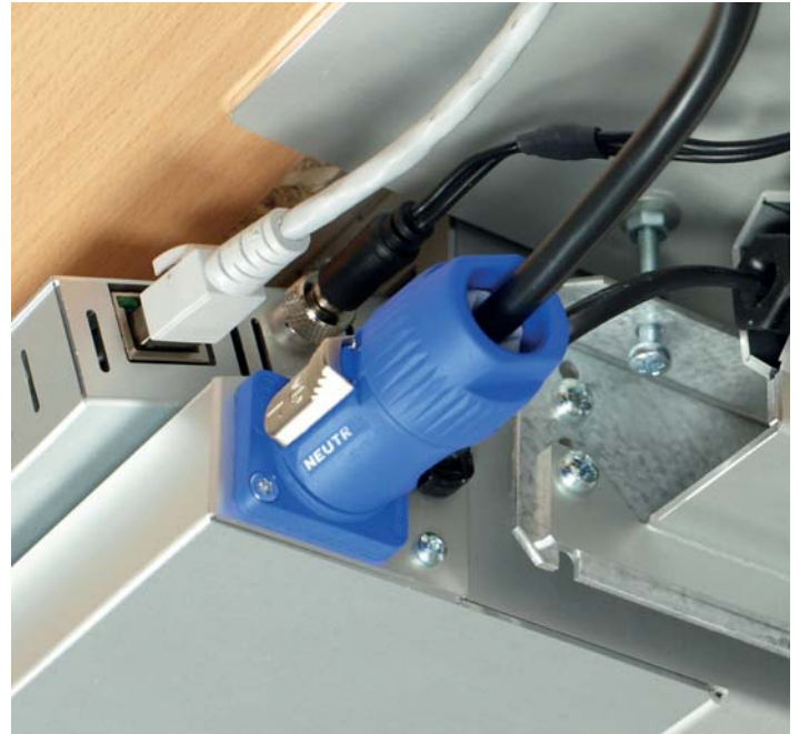
Here you can see the needed connections between the connector panels.
